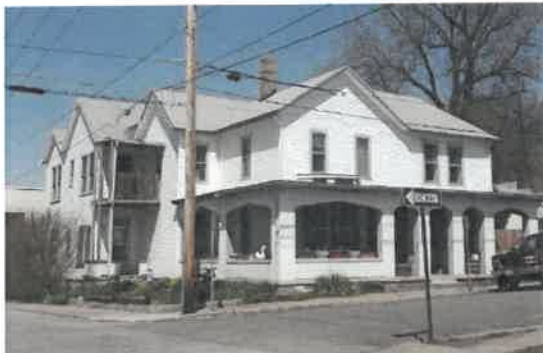
View of the current inappropriate front porch. Note how the change of roof, columns, and railings has significantly changed the appearance of the house. (STRATA)
