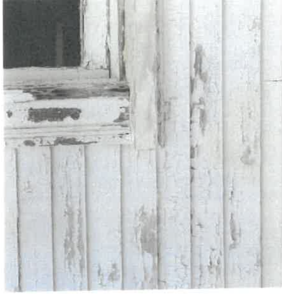
Example of deteriorated wood siding, windowsill, and trim. (STRATA)
